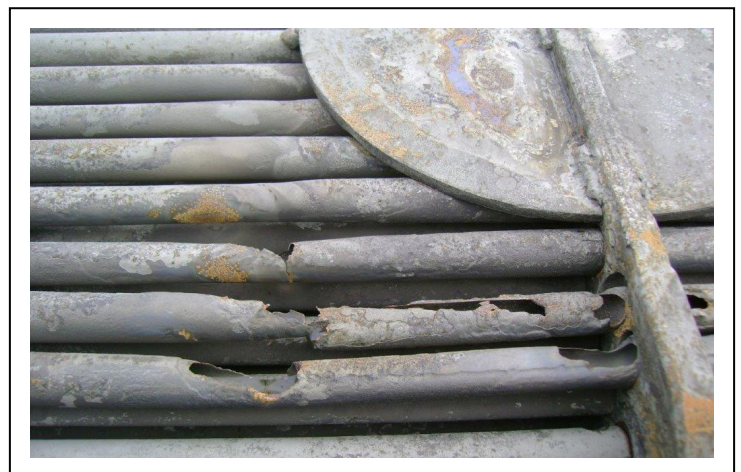
Figure 1 - Corroded heater tubes.
